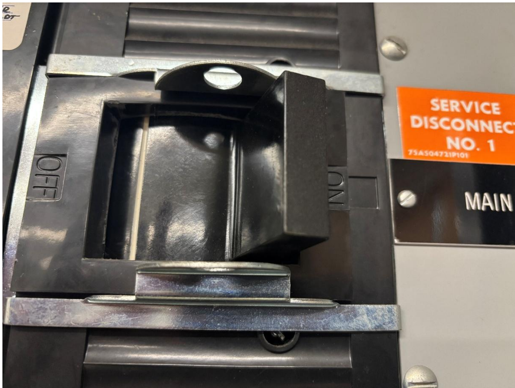
Figure 7-11. Circuit Breakers with Locking Provision
